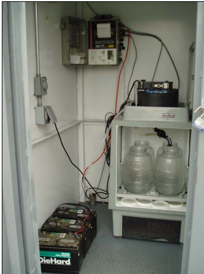
Figure 1: ISCO 6712 refrigerated sampler, ISCO 4230 flowmeter, and steel enclosure at Mass Emission site ME-VR2
