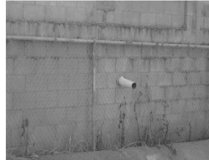
Example of an Illegal Connection
